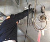
Flue Gas Temperature and Compositions Measurement
