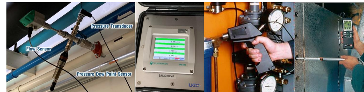
Compressed Air Flowmeters + Pressure Sensor + Pressure Dew Point Sensor with Data Loggers for Dry Compressed Air
